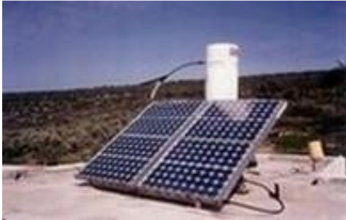
Multi Solar System, MSS Millenium Electric, Israel
